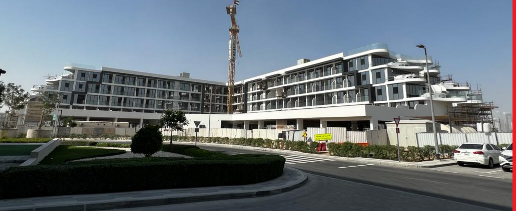
Samana Golf Avenue Residential Buildings (G+4), Dubai | Client : M/s. Samana 1 Holding Limited
